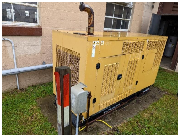
Figure 11 Existing Diesel Generator Providing Lighting Power to Motor Pool During Outages
