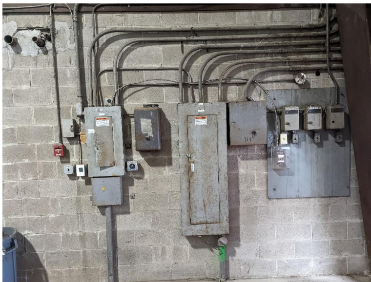
Figure 10 Bus Barn Electrical Room
